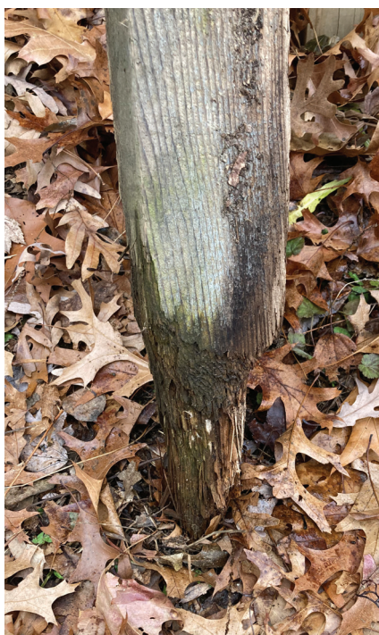
Treated post rotted at the ground line. PHOTO BY JACOB PRATER.
