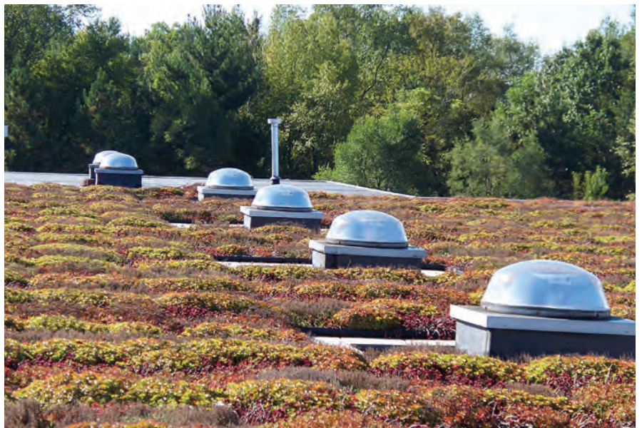
Solatube natural lighting tubes incorporated into a living roof system. PHOTO COURTESY OF KINGSPAN LIGHT + AIR NORTH AMERICA
