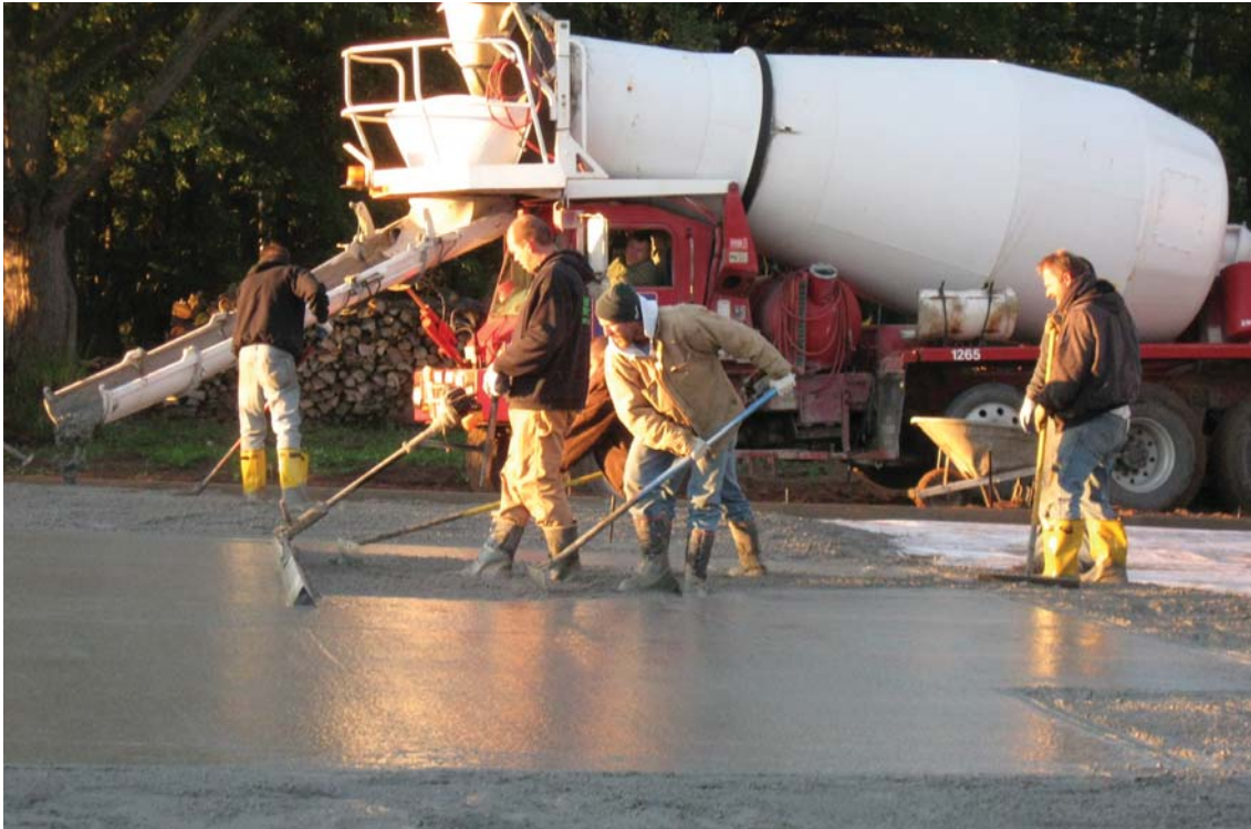
The foundation is laid for a good year, just as this concrete crew lays the foundation for a large storage shed. Rural Builder photo
