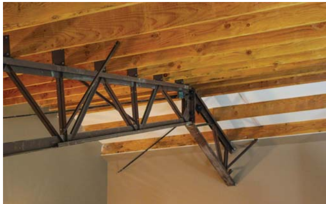
Metal meets wood in a hybrid, as shown in this inside close-up of the ceiling showing steel trusses and wood purlins. Perka Building photo.
