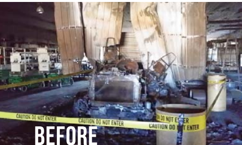
The fire didn't totally destroy the building, but damage was significant enough to cause the business to cease production for several months. Integrity photo
