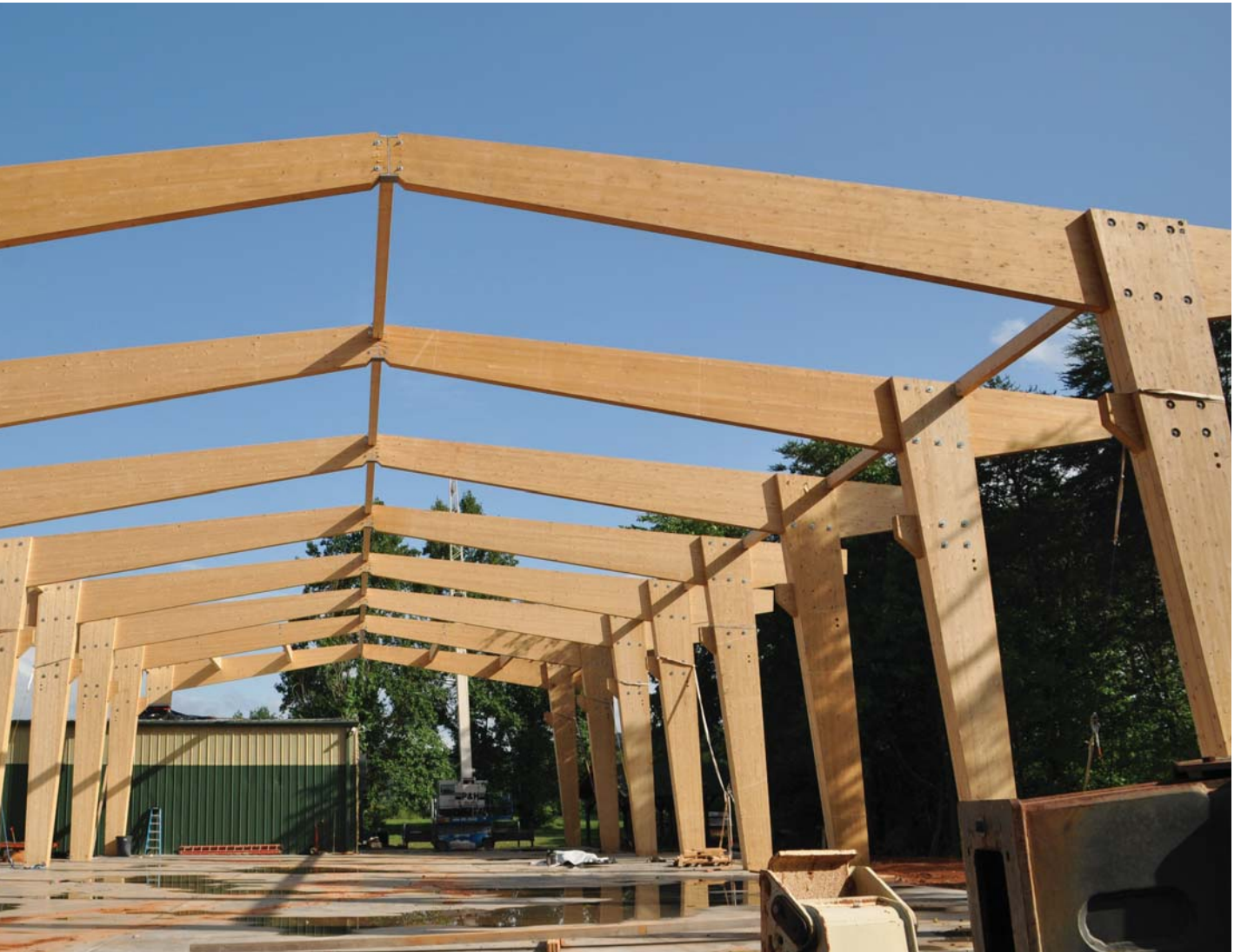
The building takes shape with each section, or bend, in place, ready for CLT wall installation. Walls were installed in pre-cut panels, five high. Sauter photo
