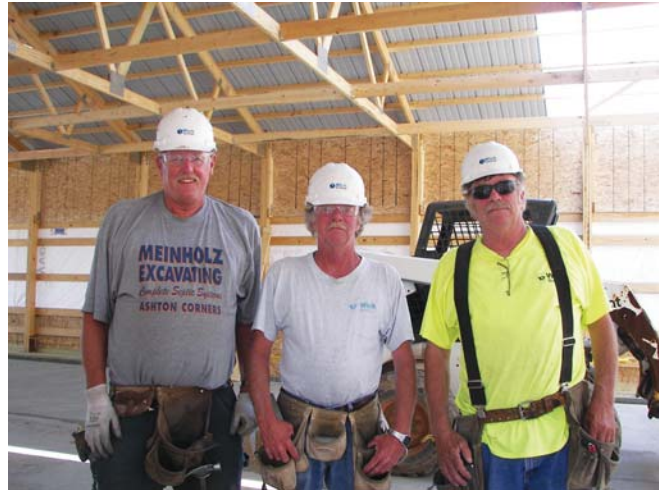
Crew members with a long and established history with a company are an increasingly rare and valued resource. Found on one Wick Buildings job site in Merrill, Wisconsin recently were these veterans (left to right) John Boda with 46 years, and brothers Loren Powell with 39 years and Roy Powell with 43 years.
