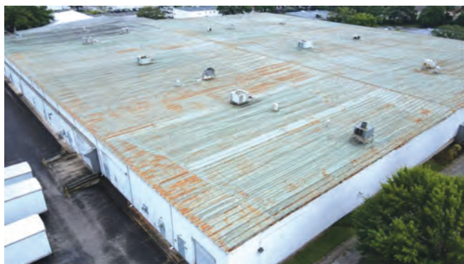
Figure 1. Before. Twenty thousand square feet of weathered standing-seam metal with rust bleed at the fasteners. PHOTOS COURTESY OF EPDM COATINGS
